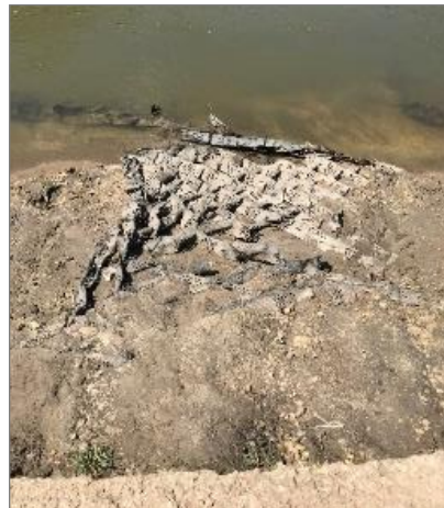
WASHED OUT SECTION AT END OF RAMP
